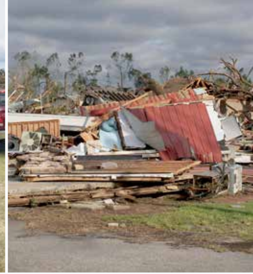
The Meat Hook, a deer-processing operation and meat market in the Moss Community of Jasper County was reduced to a pile of rubble. (Photo by Mark Thornton, Laurel Leader-Call )
